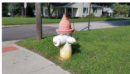
Orange Hydrant Top 500 to 999 GPM Flow Capability (Not Yet Repainted)
