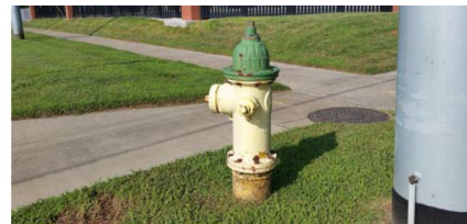
Green Hydrant Top 1,000 to 1,499 GPM Flow Capability (Not Yet Repainted)
