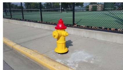
Red Hydrant Top Less Than 500 GPM Flow Capability
